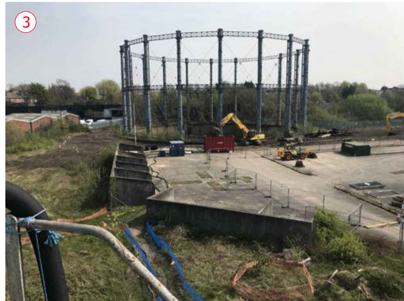
Gas holder 2 structure- since been demolished. Only base of metalwork remains and circular pit
